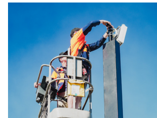
Innovation GemLife 5G Wireless Network by GemLife and Prospecta Utilities
